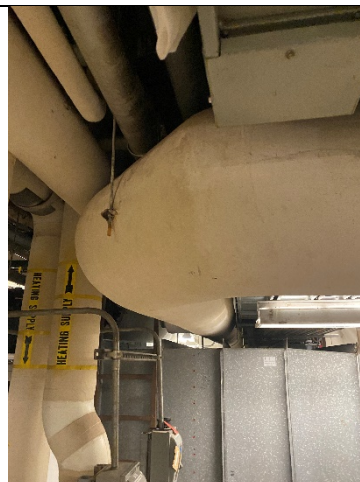
Large Diameter Vent Pipe Associated with Boiler Units
