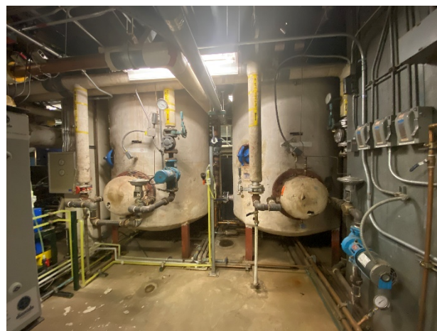
Domestic Hot Water Tanks Scheduled for Removal and Replacement
