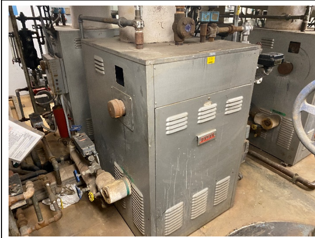
Boiler Unit Closeup
