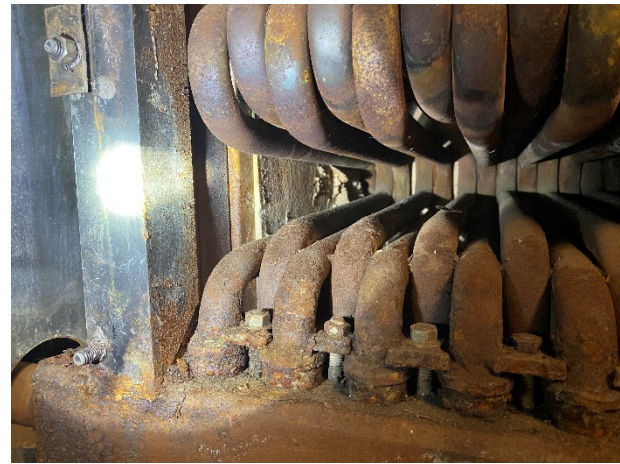
Boiler Unit Closeup Interior – White Fibrous Insulation Visible
