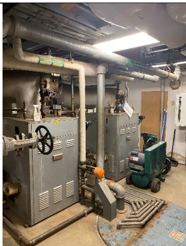
Typical Boiler Units Scheduled for Removal and Replacement
