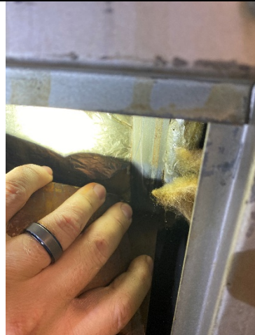
Boiler Unit Closeup Interior – Fiberglass Insulation Visible
