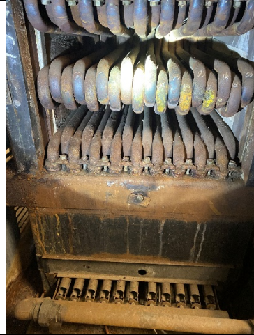
Boiler Unit Interior
