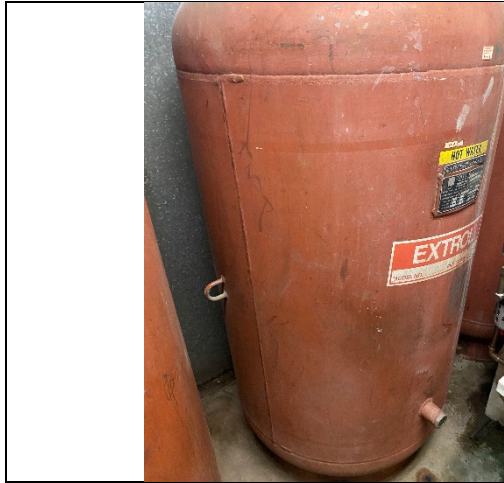
Chiller / Heater Tanks
