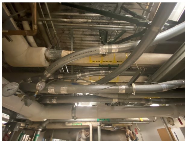
Typical Ceiling Level Piping
