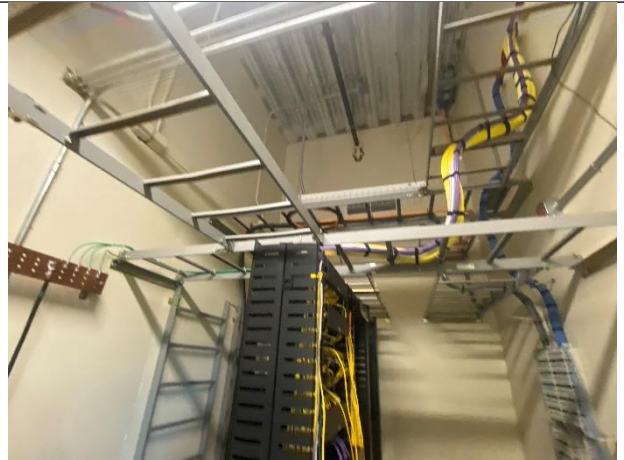
View of the ceiling in one of the telecom rooms
