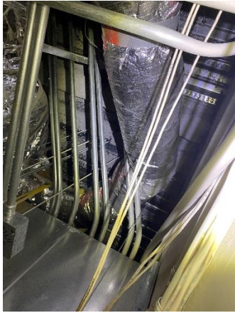
View above the ceiling tile in the adjacent corridor of one of the telecom rooms
