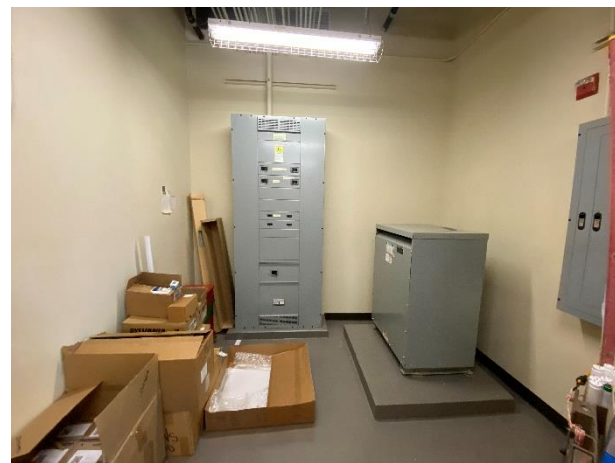
Additional view within one of the other telecom rooms
