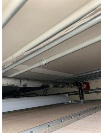
View above ceiling showing uninsulated pipes
