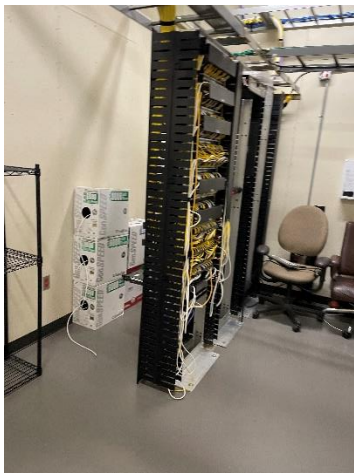
View inside one of the telecom rooms
