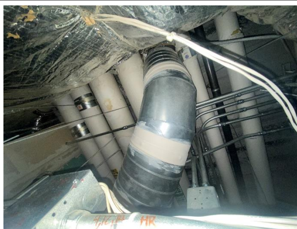
View above ceiling showing fiberglass insulated piping and HVAC ducting
