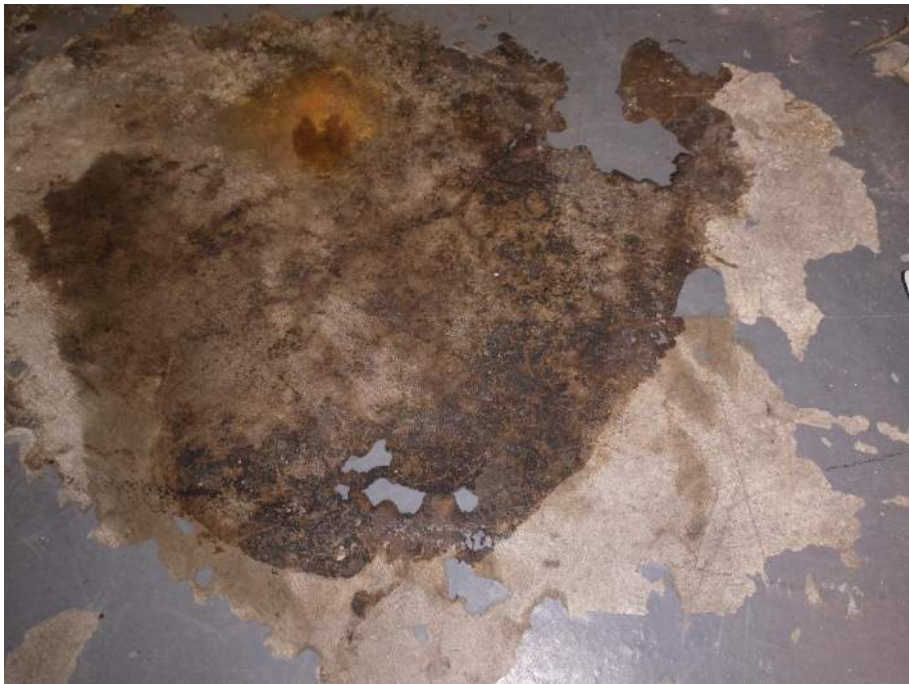
Closeup of washed floor area with delineation between visible and non-visible black mastic
