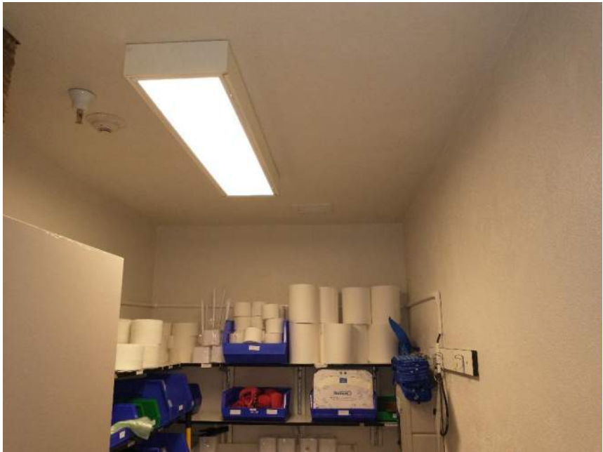
8 th Floor Janitor Closet 8122 with rough plaster walls and ceiling
