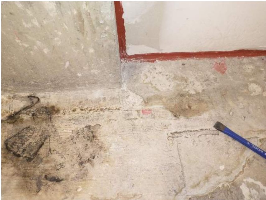
1 st Floor Vacant Space 1119 with visible black floor mastic post wash
